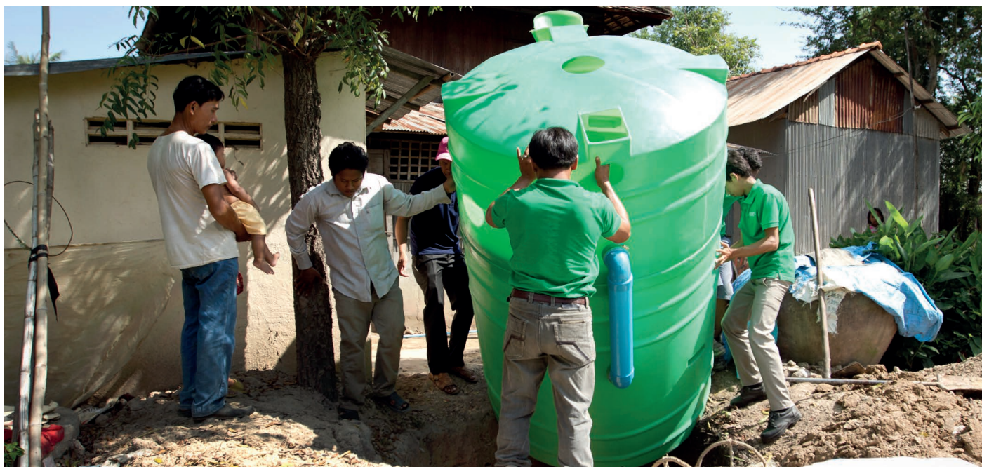
INSTALLATION OF AN ATEC BIODIGESTER IN CAMBODIA. The biodigester was designed for floodplains, replacing traditional firewood based cookstoves while also producing bioslurry as fertilizer. The use of the biodigester can save farmers up to US$521 per annum while also reducing carbon emissions and deforestation. Photo: ATEC
