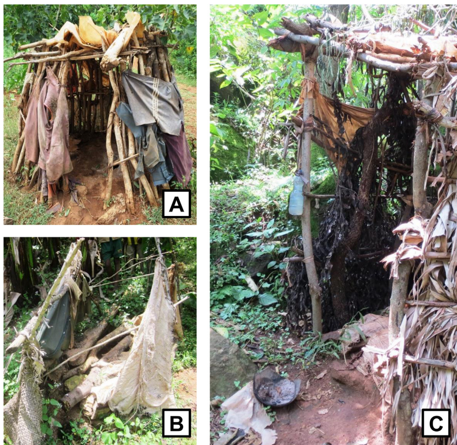
Fig. 1. Examples of typical sanitation facilities. A – Pit latrine ensuring some privacy, apparent footpath, solid slab, no cover; B – Collapsed latrine; C – Pit latrine with water and ash available for handwashing.
