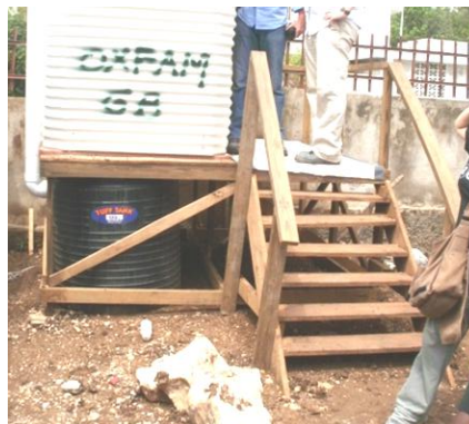
Figure 6.21 Single compartment holding tank
