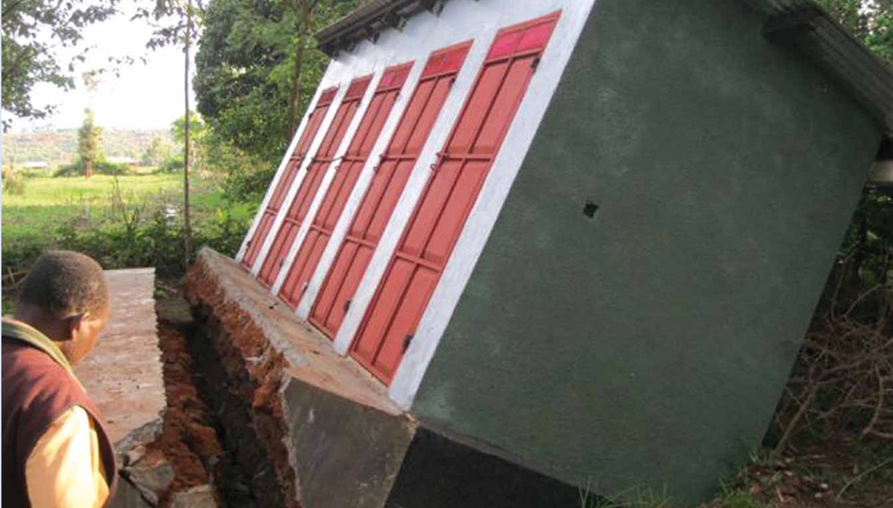
Collapsed School Toilet Building after Heavy Rains (Photo: Source unknown)
