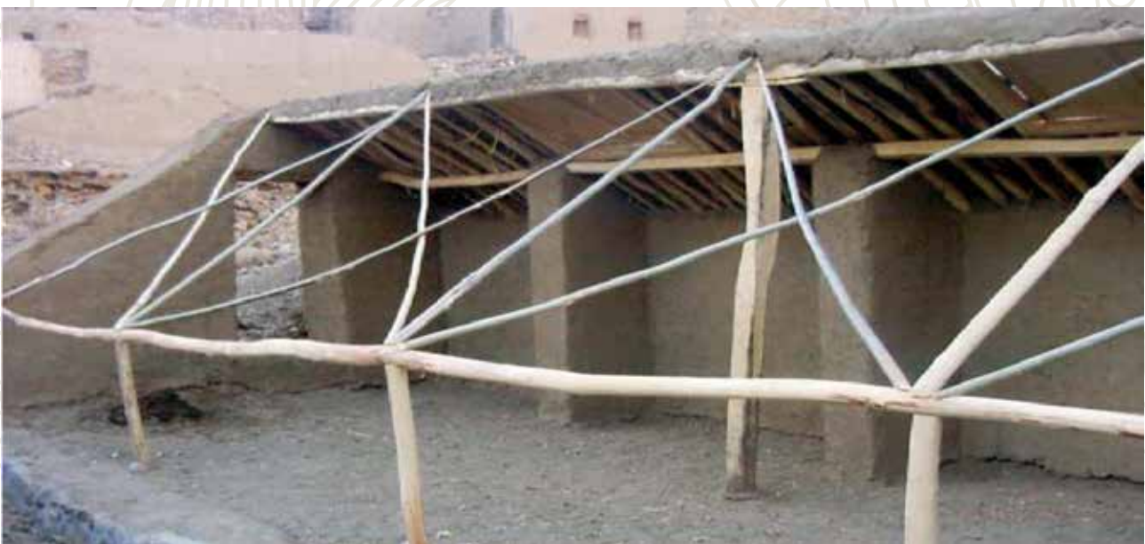
Picture No. 10: The inner construction of the greenhouse – main horizontal beam supported by wooden slope and the second horizontal beam supported by the partition north walls
