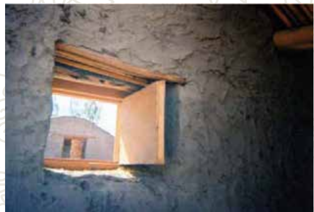
Picture No. 7: Installed wall ventilator
